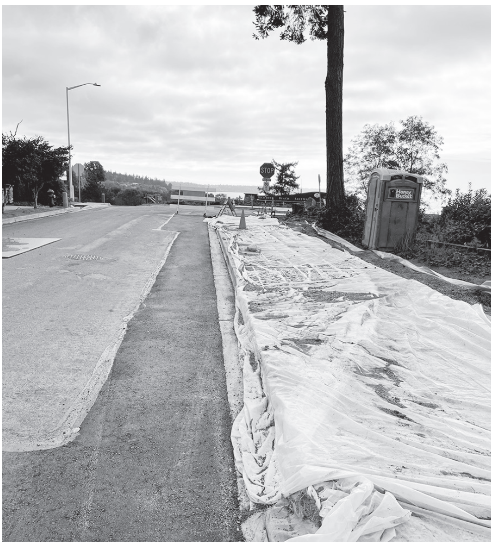
VIEW OF THE NEW SIDEWALK CONSTRUCTION LOOKING SOUTH TOWARD RICHMOND BEACH SALTWATER PARK ON OCTOBER 20.
