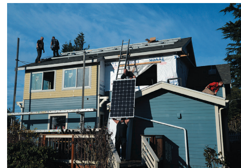
SOLAR PANELS GO UP ON THE SOUTH SIDE OF THE HOUSE, NOVEMBER 25, 2013
