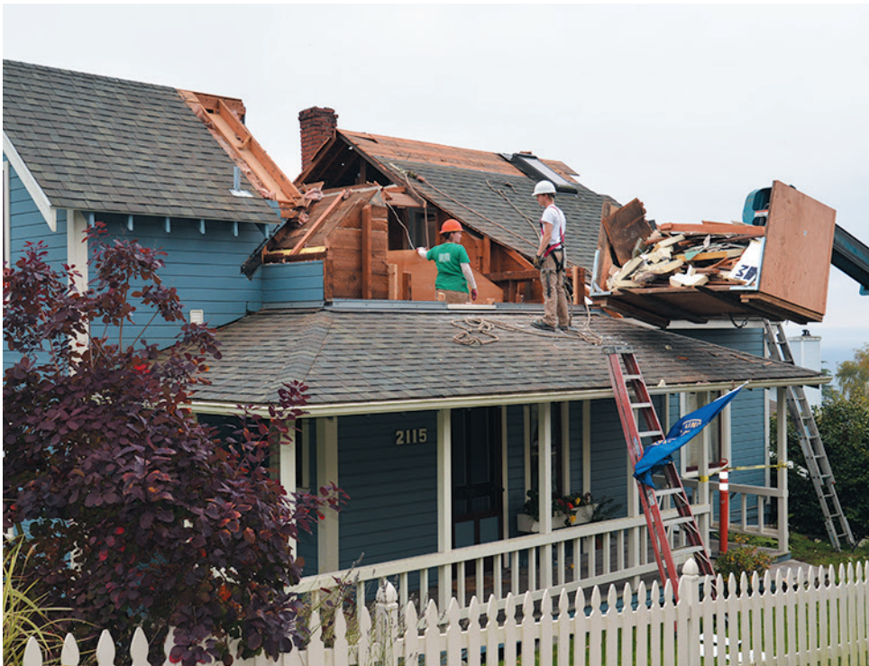
THE NORTH GABLE COMES OUT, OCTOBER 16, 2013 -ALL RENOVATION PHOTOS ON PAGE 4 BY RICHARD W. CLARK
